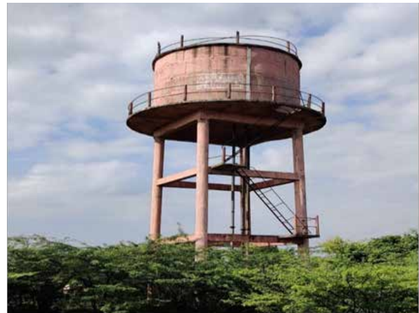
Figure 2 Elevated service reservoirs
